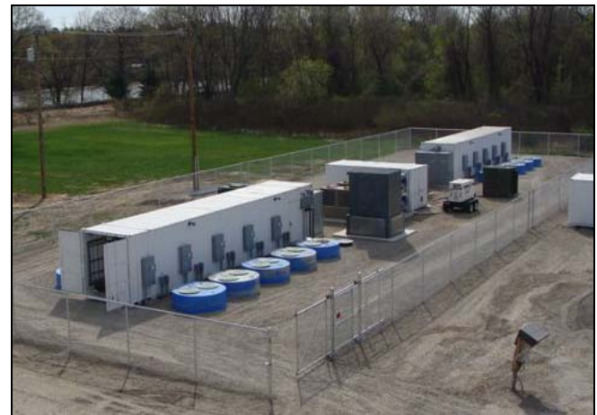
Figure 7. Two MW Beacon Power flywheel storage in frequency regulation service in ISO-NE
